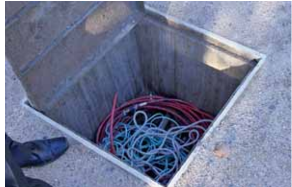
Exterior cable pit with pull-through.
