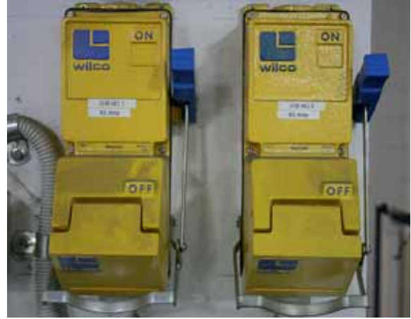
2 x 63 Amp Wilco 3-phase outlets.
